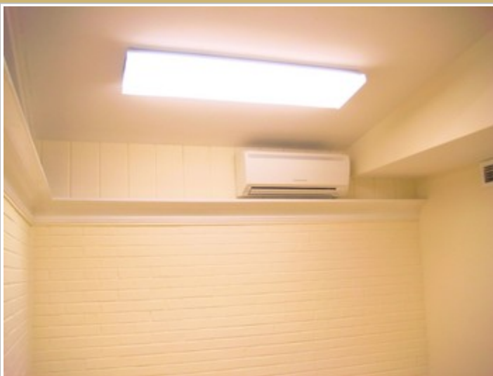
Office 2 - Additional Mitsubishi HVAC U
